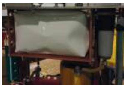
Oil protection of an electrical power transformer
