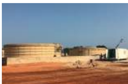
BOLTED FUEL TANK
