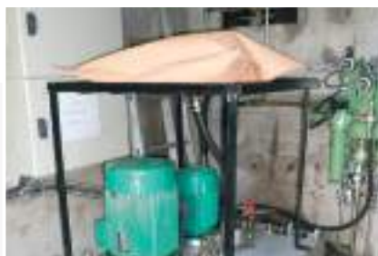
Lock gate motor oil protection Hydraulics
