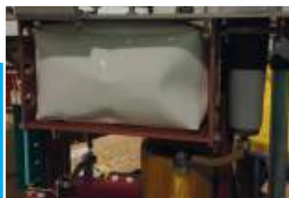
Protection of transformer oil - Electric -
